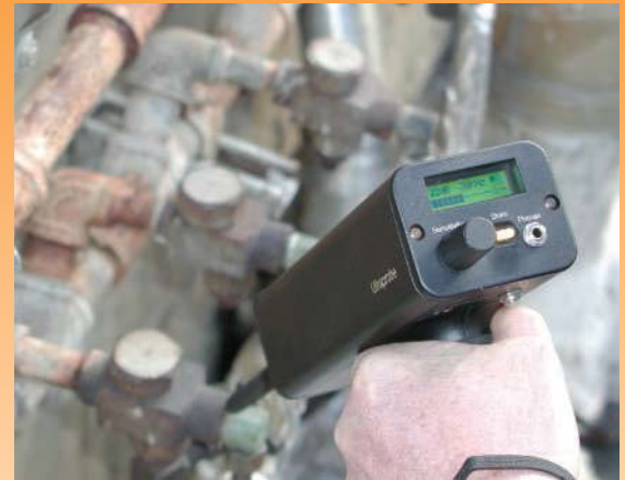
Inspect steam traps
